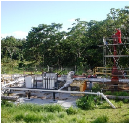
Remote Amazonian LPG terminal needs valve repair.
