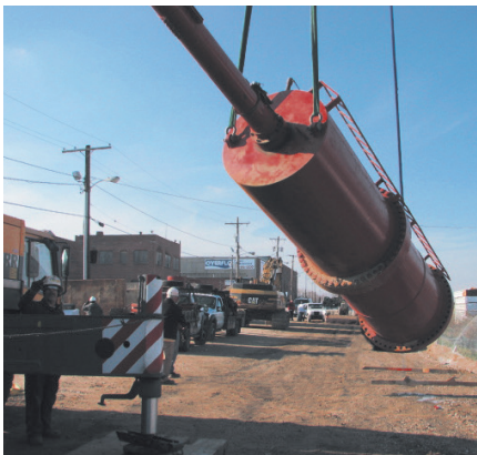
TDW acts to repair the city of Baltimore's decomposing primary wastewater collection line.
